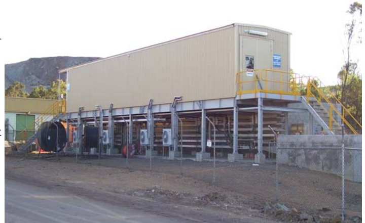
SSIA—new substation completed
