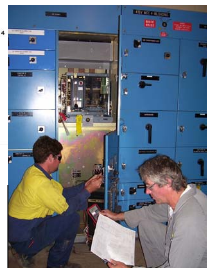
O'Donnell Griffin commissioning crew, Craig Valmadre and Peter Warry, at Substation 3
