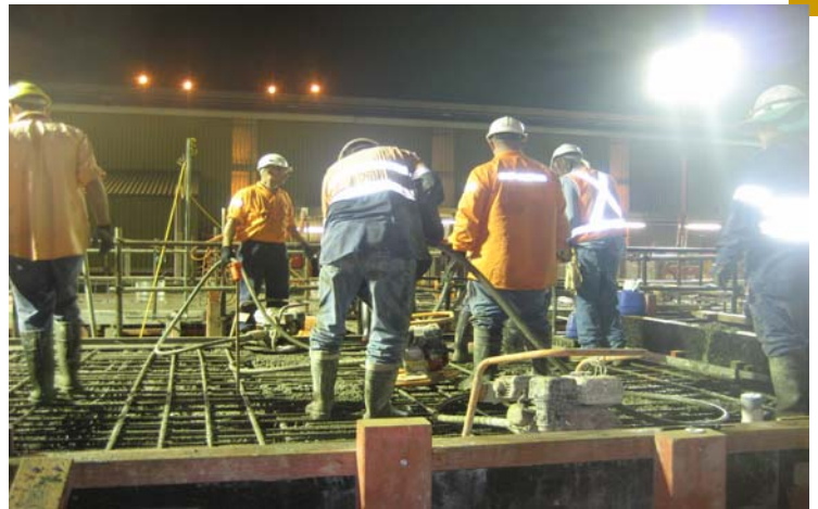
An impressive 240m 3 was poured, starting at midnight on the Rail Receival Pit
