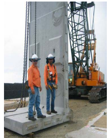
BMD rigger/operator Chris Zammit, Rigger Phil Simon, and Walter Wright crane operator Graham Youngberry manoeuvre the first of over 1100 concrete wall panels that will form the vertical walls of Bund 5A into position.
