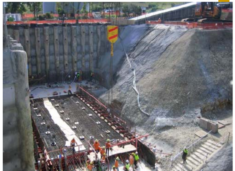
Excavation complete! Concrete works in the Rail Receival Pit has now commenced
